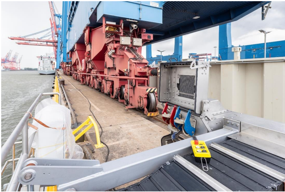
Figure 19: Moveable HV shore connection Port of Hamburg - Copyright HPA / Schmidt-Wiethoff
